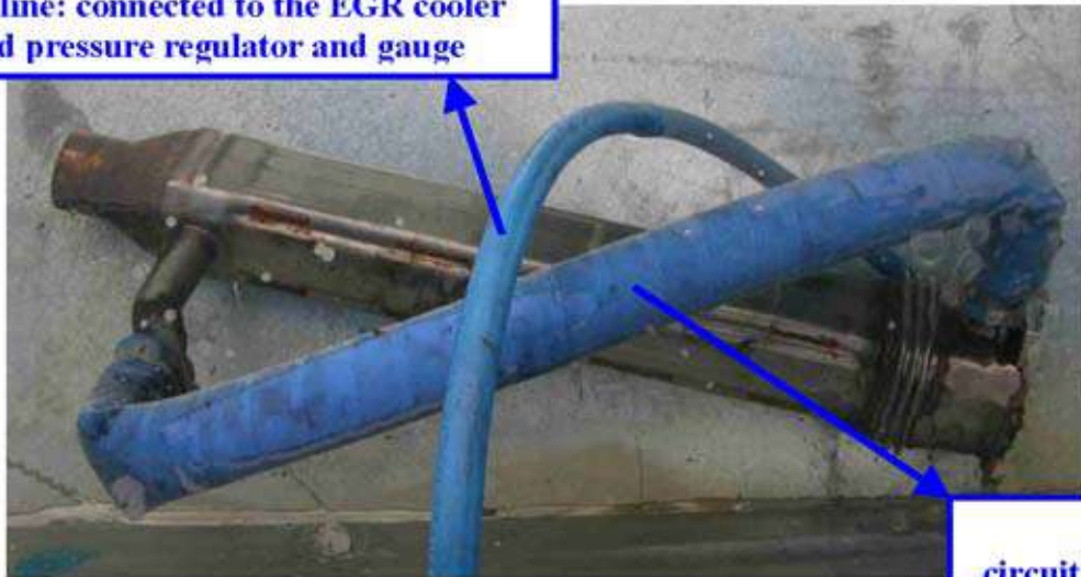
Figure 2 - EGR cooler ports: short-circuited
